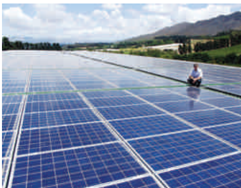
Clemens Brandt of RED Engineering admires the nearly 3000 m 2 extent of the solar panel installation at Arbeidsvreugd in Villiersdorp. PHOTO: NICK YELL
