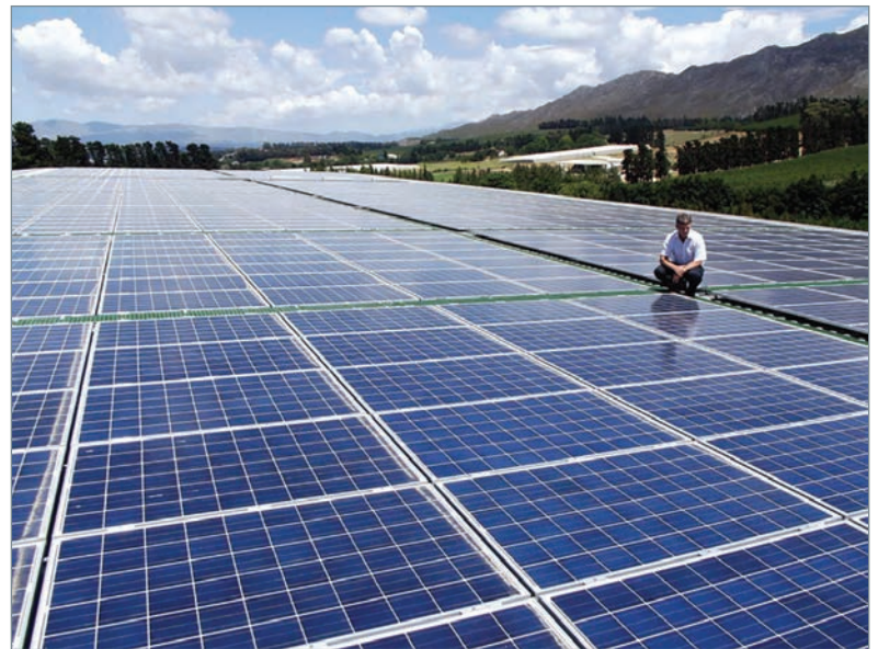
Clemens Brandt of RED Engineering admires the nearly 3,000m 2 extent of the 1876 solar panel installation at Arbeidsvreugd in Villiersdorp.
